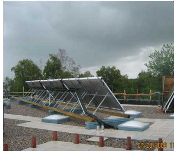
Figure 4: Solar Hot Water on roof of new Water Plant
