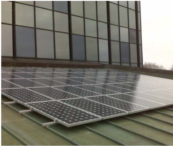
Figure 3: Solar PV on roof of City Hall
