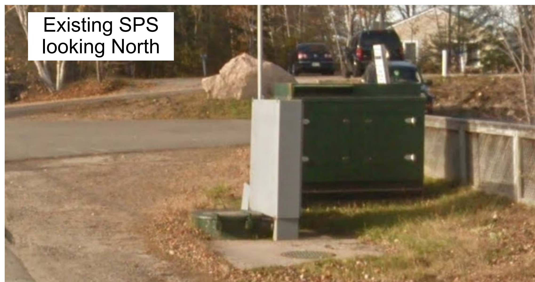
Premier Road Sewage Pumping Station, Forcemain and Sanitary Sewer Class Environmental Assessment
