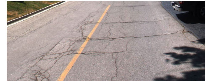
Poor Road Condition
