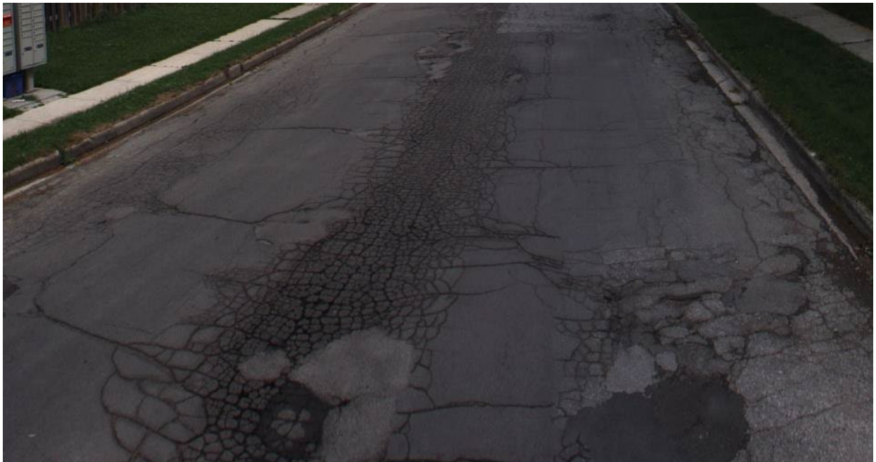
Very Poor Condition
