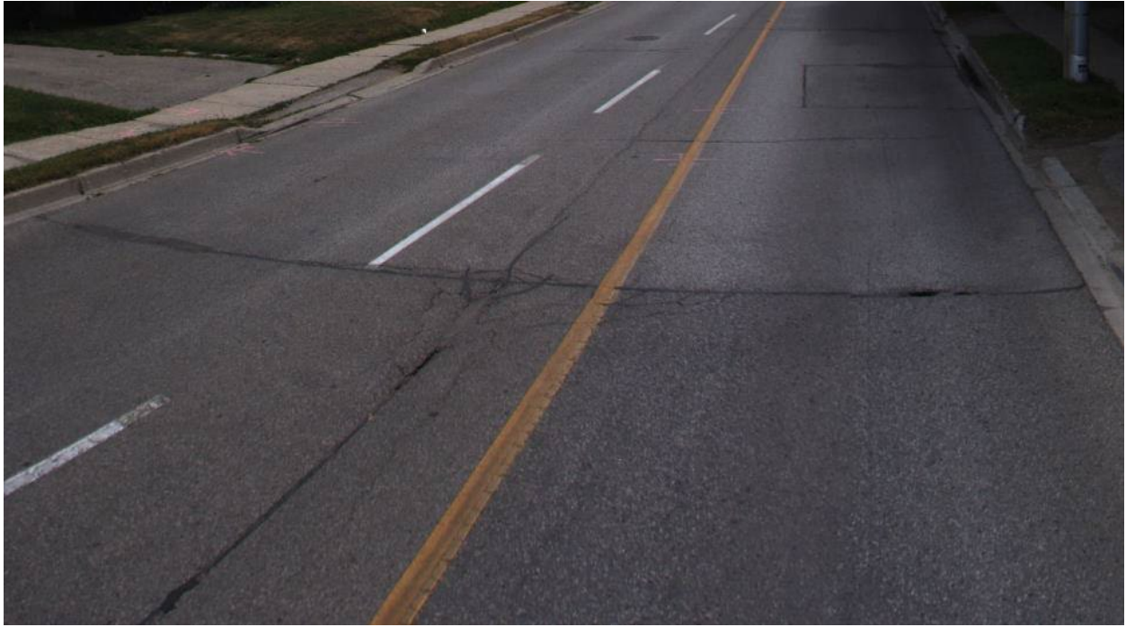
Fair Road Condition
