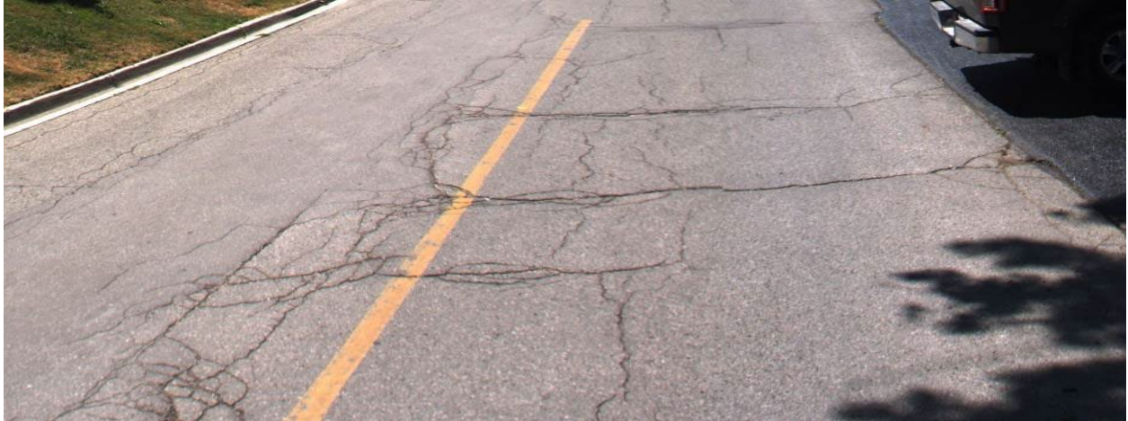
Poor Road Condition
