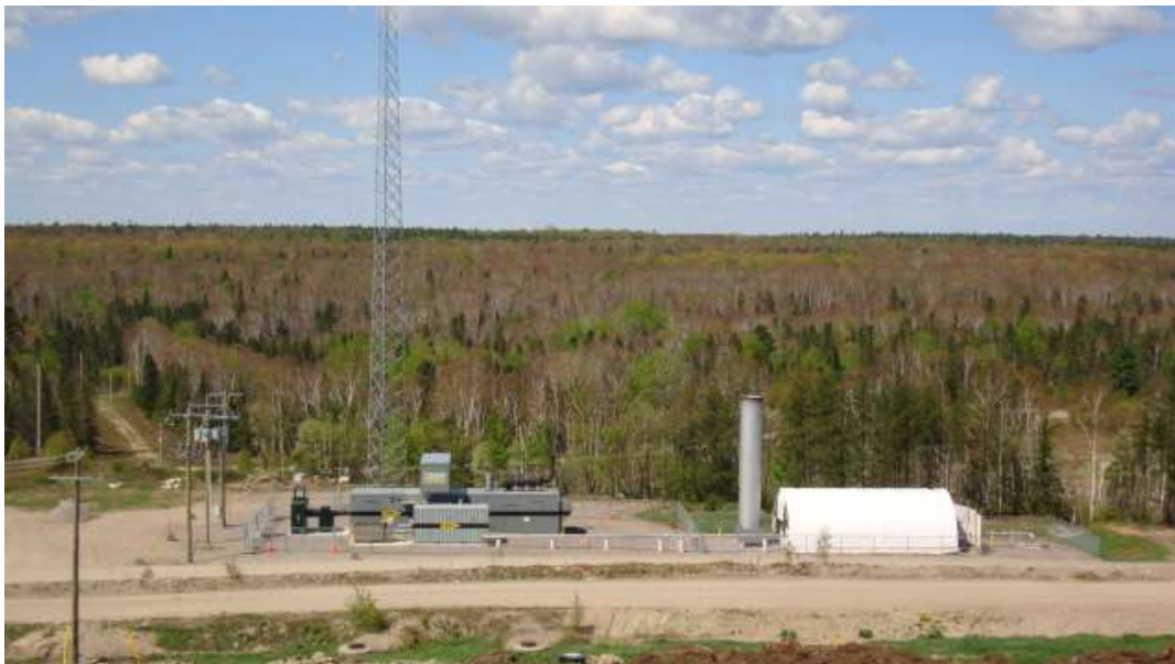
Figure 4: Landfill Gas Utilization to Electricity Facility and Landfill Gas Flaring Station located at the City's Merrick Landfill Site
