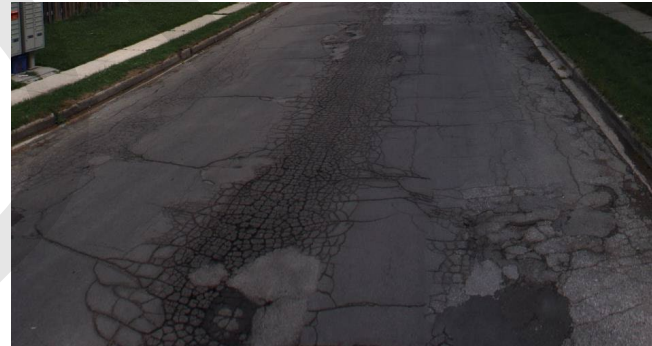
Very Poor Condition
